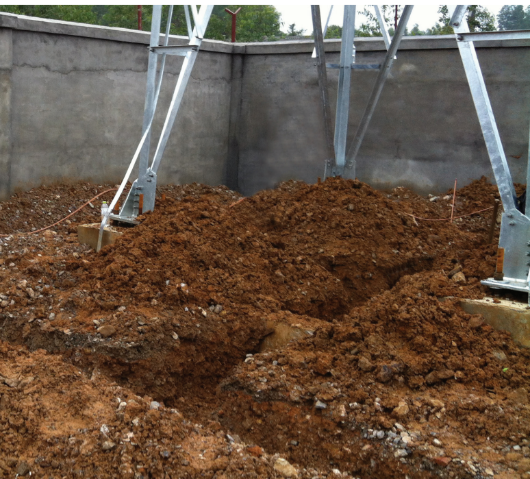
Telecom tower grounding
