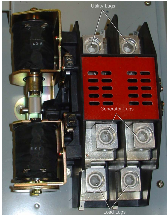
Figure 11. Cable Connection Locations (200 A).
